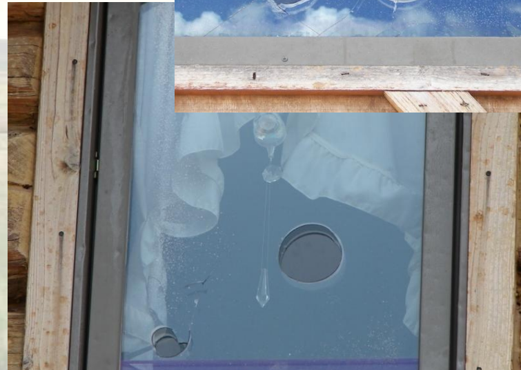
Hail Damage on May 22, 2008 (Courtesy of Jeff Mitros)
